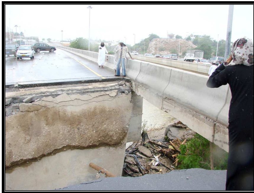
Photo 1: the damaged part of the bridge
